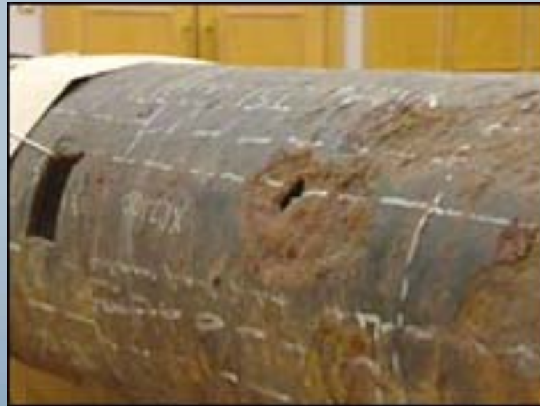
Corroded ductile iron gas pipe.
