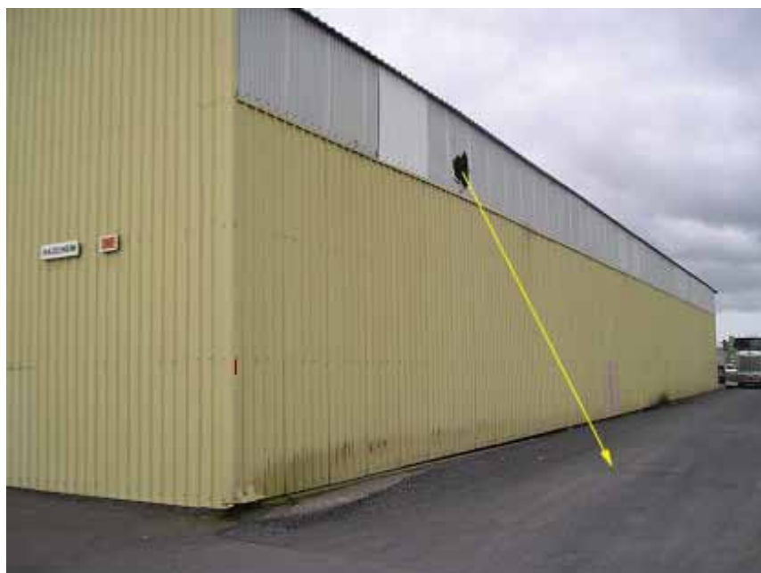
Photo of the hole made by the extinguisher as it exited the building and the landing area to demonstrate the distance flown and force of the escaping gas.
